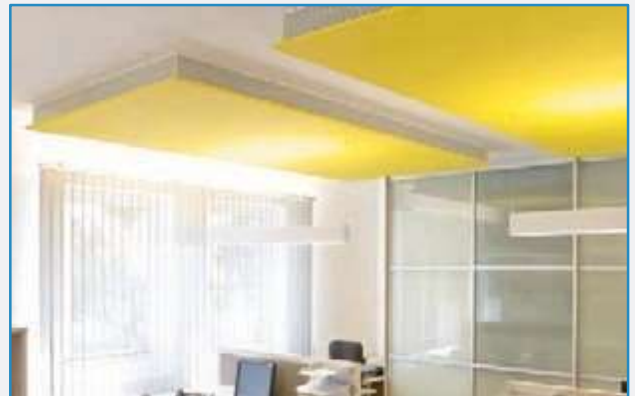
▲ Example of a "ceiling sail"
